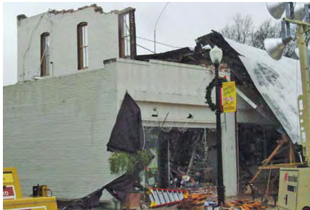
Collapsed roof in downtown Paso Robles following the San Simeon earthquake of December 22, 2003. Two people were killed by falling debris when they ran out of the building. (USGS photo)
