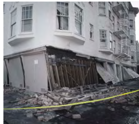
“Soft story” buildings, typically with parking on the ground floor, like the one pictured here, are common throughout the Bay Area and are particularly at risk when exposed to strong shaking (USGS photo).
