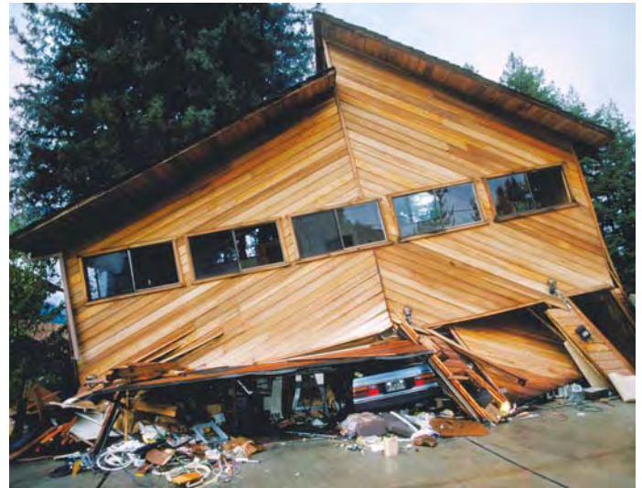
This home in the Santa Cruz Mountains collapsed in the 1989 magnitude 6.9 Loma Prieta earthquake (USGS photo).
