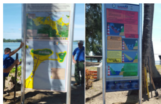
Figure 2. Tsunami signs installed at very visited beaches
